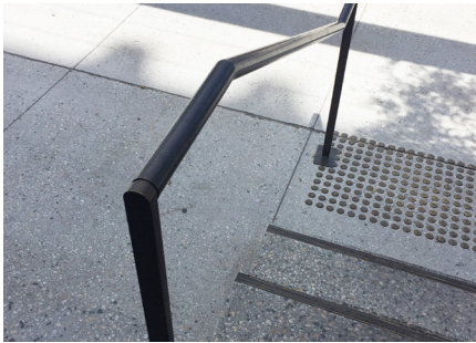
Black Powder Coated Handrail
